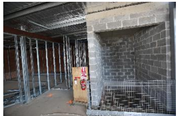
Figure 6: New meeting rooms framed up and lift well ready for fit out
